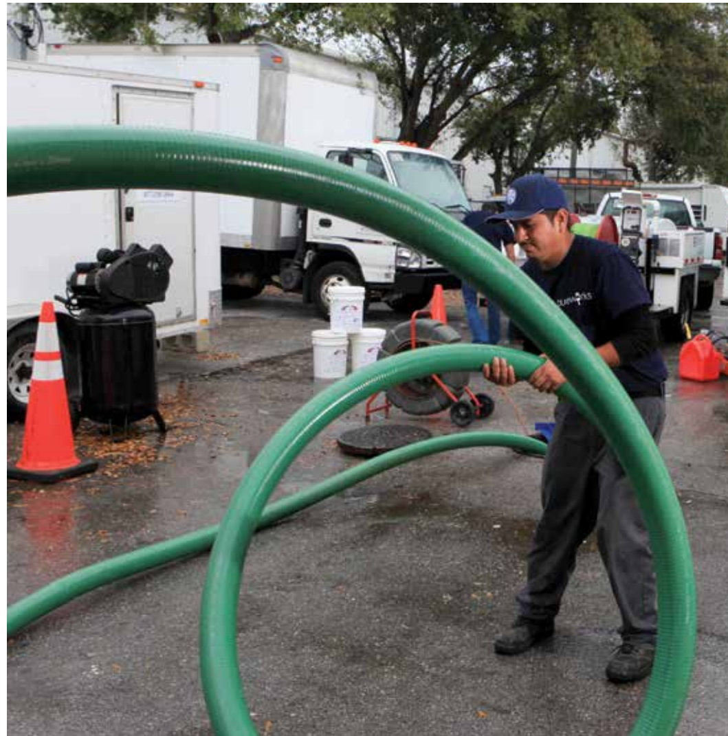
Eric Pinto uncoils a vacuum hose while the crew cleans and inspects a sewer main.
